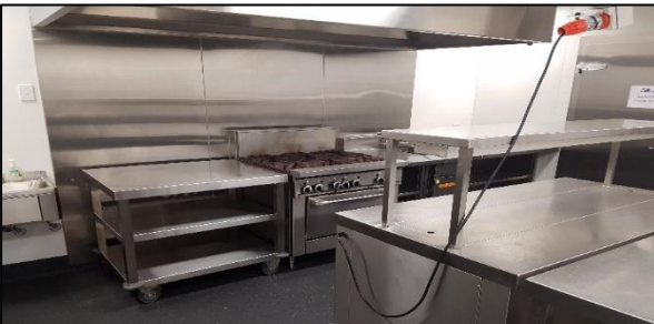
Commercial Gas Stove and oven, Deep fryer, Cool Room
